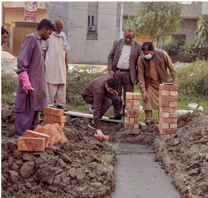
4th December 2021: CEO Zaman Foundation, Mr. Omar Zaman, breaking the ground for the construction of Marina Ali's house.
